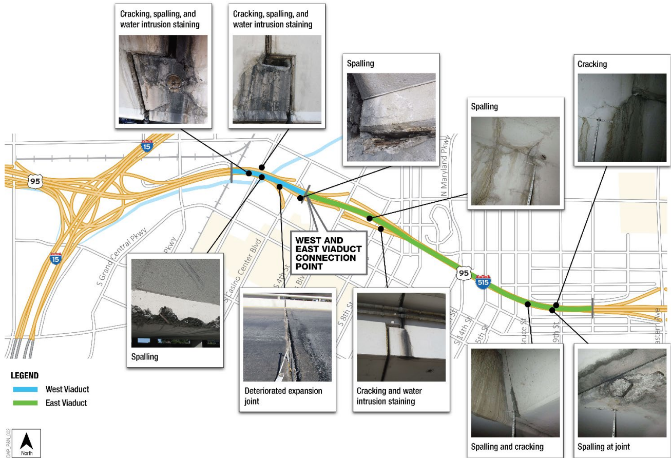
1 Figure 1-4. Viaduct Deterioration
